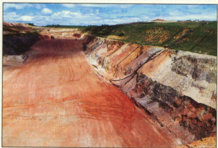
Prior to reclamation, the Flambeau Mining Co. replaced six million tons of spoil that it had removed from the 360-foot deep pit during mining. Once the surface was recontoured to replicate its original condition, Applied Ecological Services planted the site into over 10 different ecological communities.
